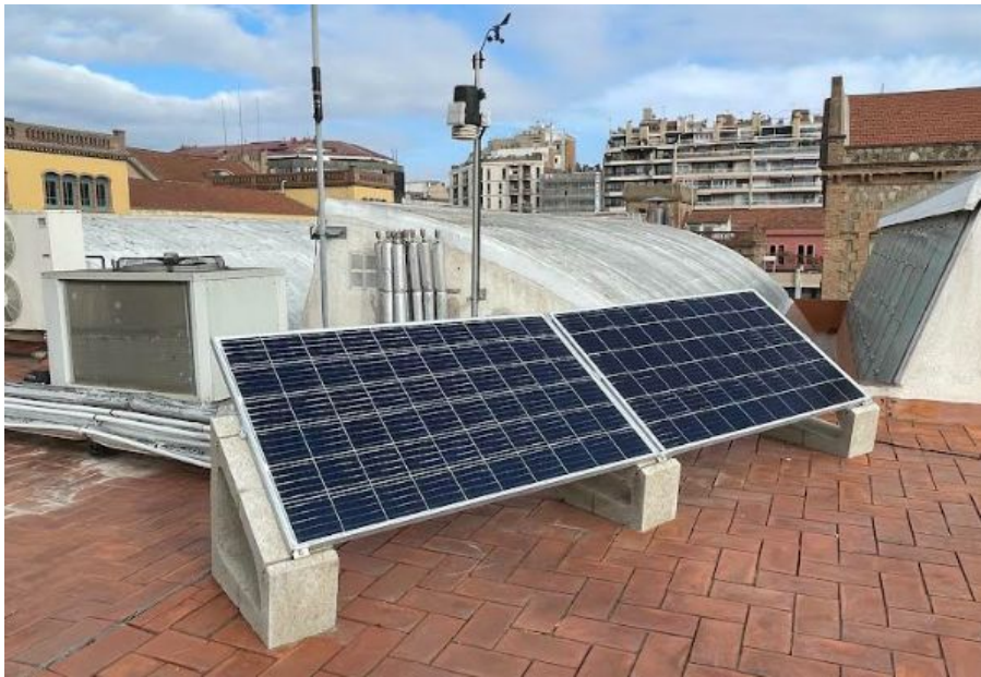
Photovoltaic panels on the roof at edt
